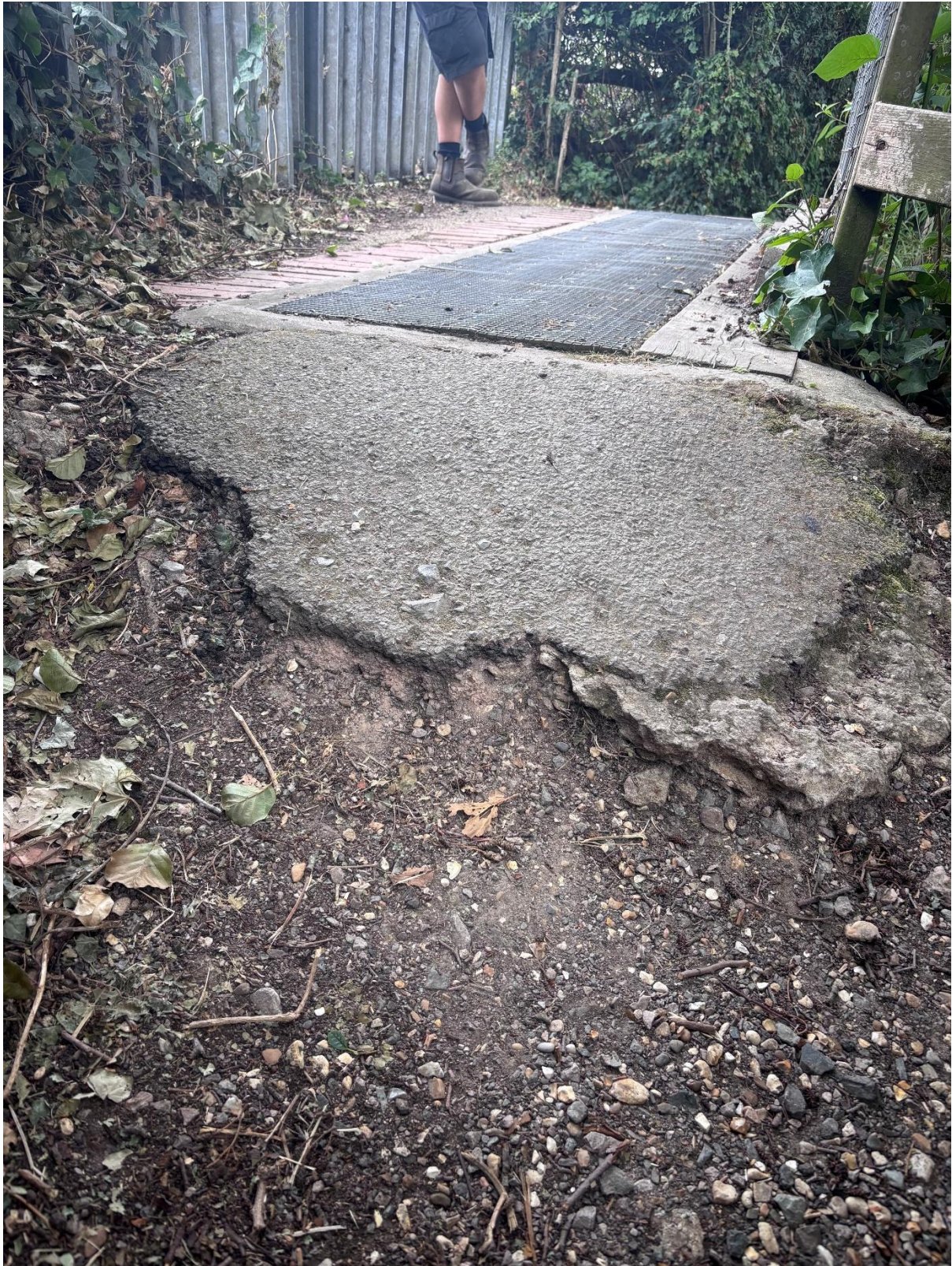
Trip hazard at the pathway, there is at least one other example of this, and also the tree roots within the pathway in another area.
